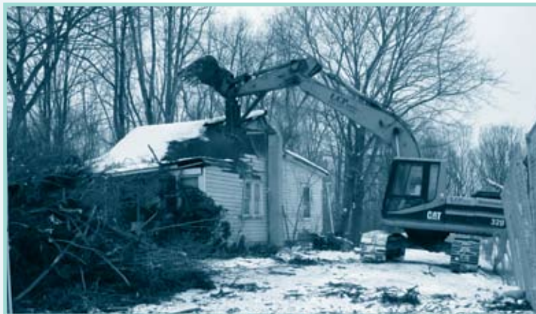
Larry Pierce of LCP is shown operating an excavator with demo claw to take down the house.
